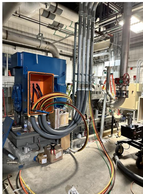
Figure 2.3.3. Magnet cooling water pump MCP1F shown during the connection of electrical services from the variable speed drive.
