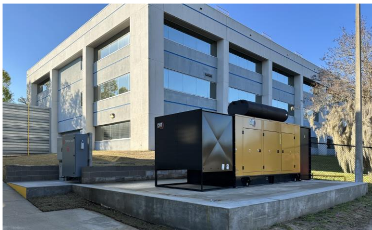
Figure 2.3.2. New 500kW Emergency Generator
