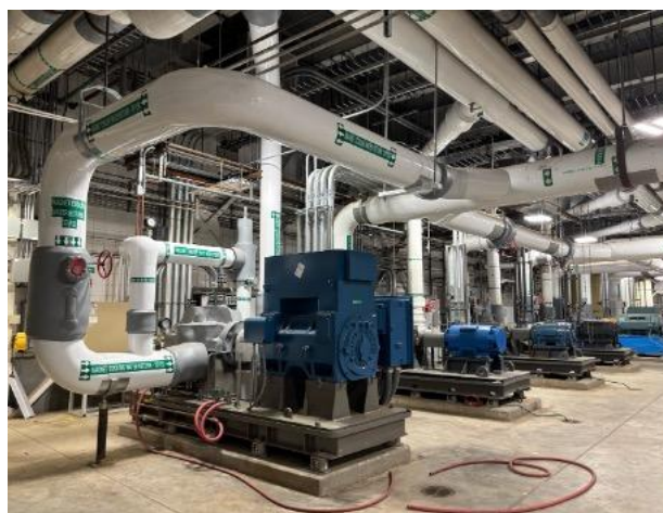
Figure 2.3.2 Primary magnet cooling water pumps and variable speed drives in the DCF water-cooling plant.
