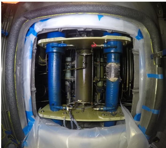
Figure 4.1.28 View of the blue SCH current leads after access panel was removed. The damaged section can be seen by the discolored section on the right 20 kA lead.
