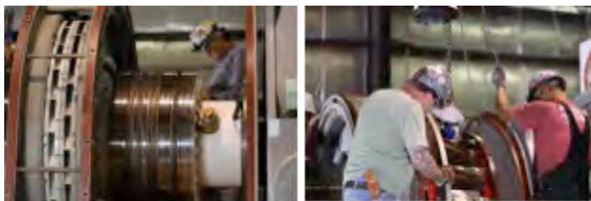
Figure 2.b.25: Work to resurface the generator sliprings and upgrade the carbon brush configuration to enable high current operation in the future.
