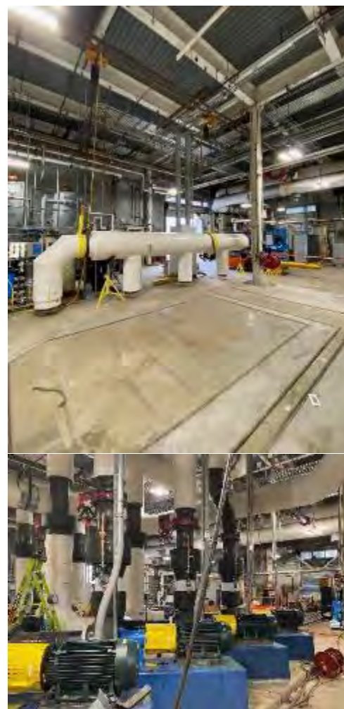
Figure 1. Top: One of the large plumbing headers prior to being lifted into place. Bottom: Four of the eight pumps set in place and in final stages of installation.
